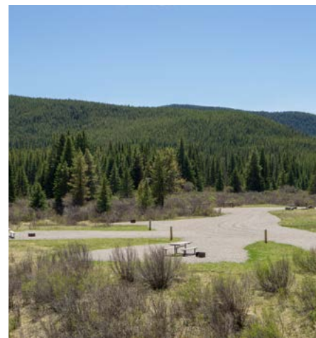
Clockwise: Clearing in-growth with a feller buncher; freshly graveled and levelled sites; new picnic tables ready for placement
